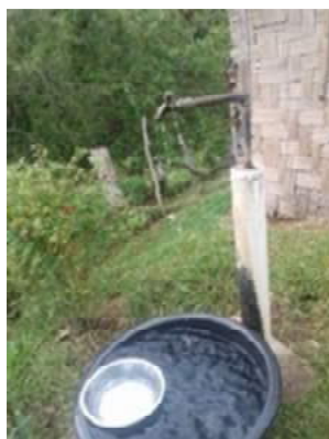
Handwashing Facility at Lalzadeth Primary School
