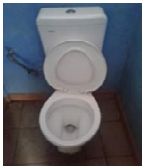
Button flush toilet at Melsisi Primary School
