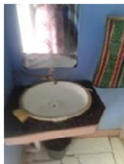
Handwashing basin at Melsisi Primary School
